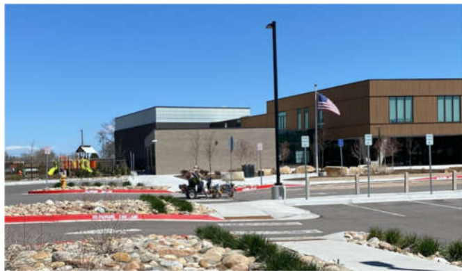
(Above)- Workers painting curbs of fire lane just north of sensor location.
